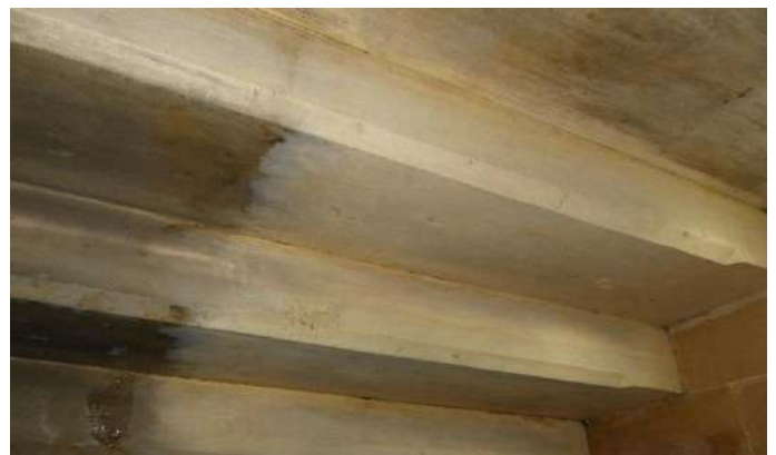
Once all of the soiling is in the gel and the surface looks clean underneath, remove the gel.
