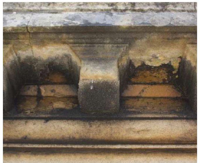
An example of sulphated limestone masonry prior to treatment.
